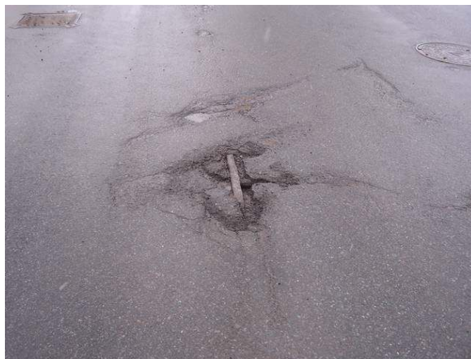
Close up of Street car rail in pothole
